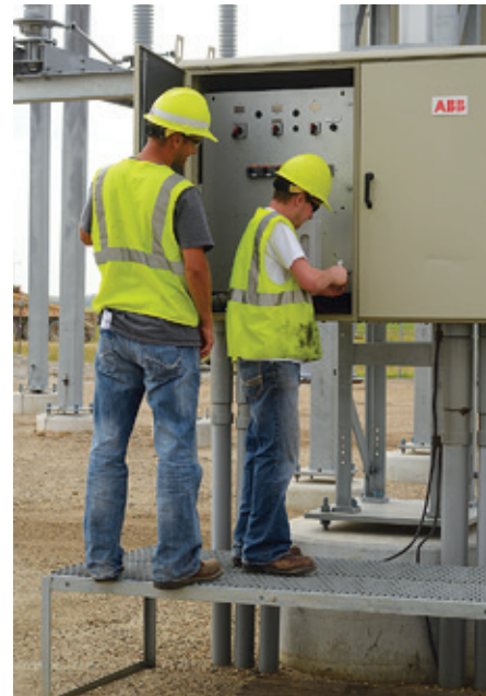
Jason Bjerke, left, technical maintenance technician, and Chris Kelley, senior technical maintenance technician, work on circuit breaker controls in the Prairie substation shortly after the line was energized for the first time.
