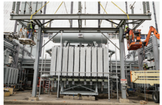
From their bucket trucks, Minnkota transmission crew members help position the new generator step-up (GSU) unit at the Young Station.
