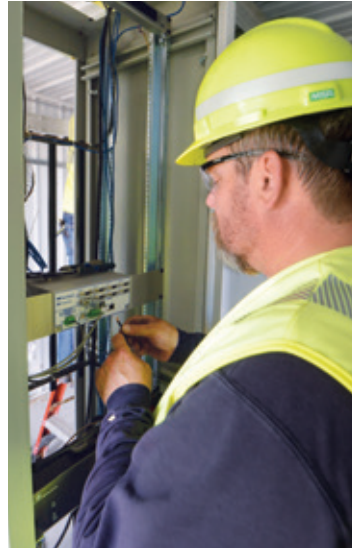
Jason Johnson, Minnkota senior technician, completes telecommunications wiring work as part of the distribution automation project.
