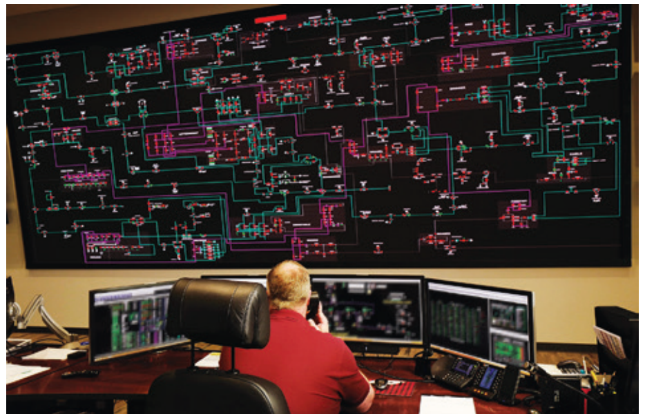
The distribution automation project will help provide Minnkota power system operations personnel like Mike Bedney with more information from substations across Minnkota’s system.
